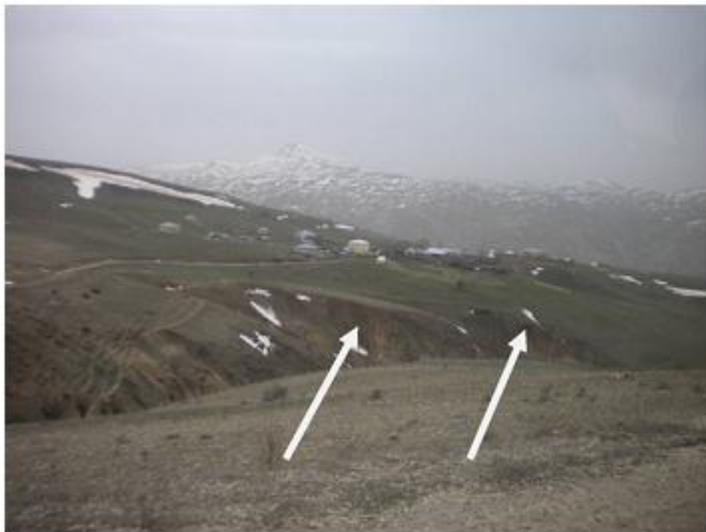
Figure 3.10 : Slope failures around the stream in the region (Celep et. al, 2010).
