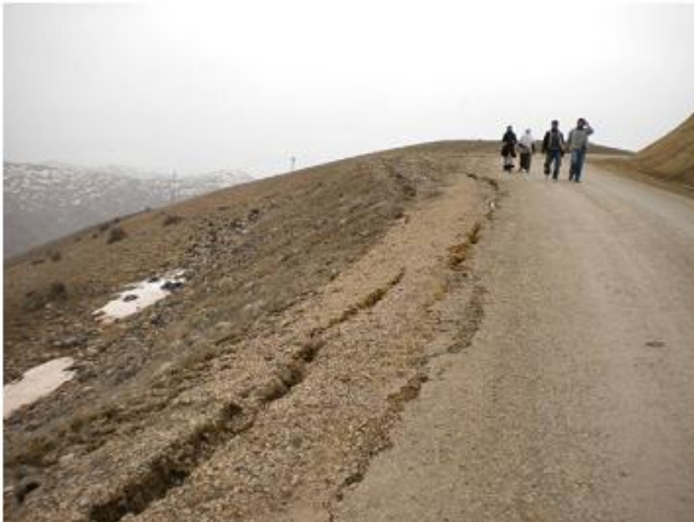
Figure 3.8 : Tension cracks on the side of the road in the region (Celep et. al, 2010).
