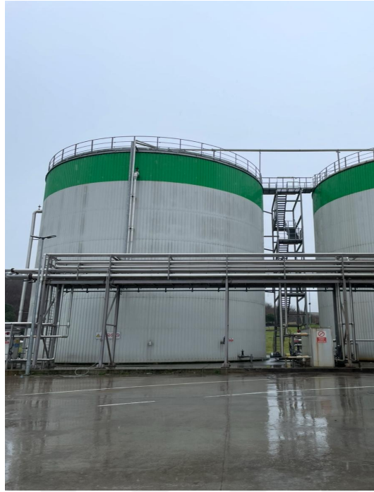
Figure 4.1. Digesters, Istanbul Metropolitan Municipality Kemberburgaz Biomethanization Plant.
