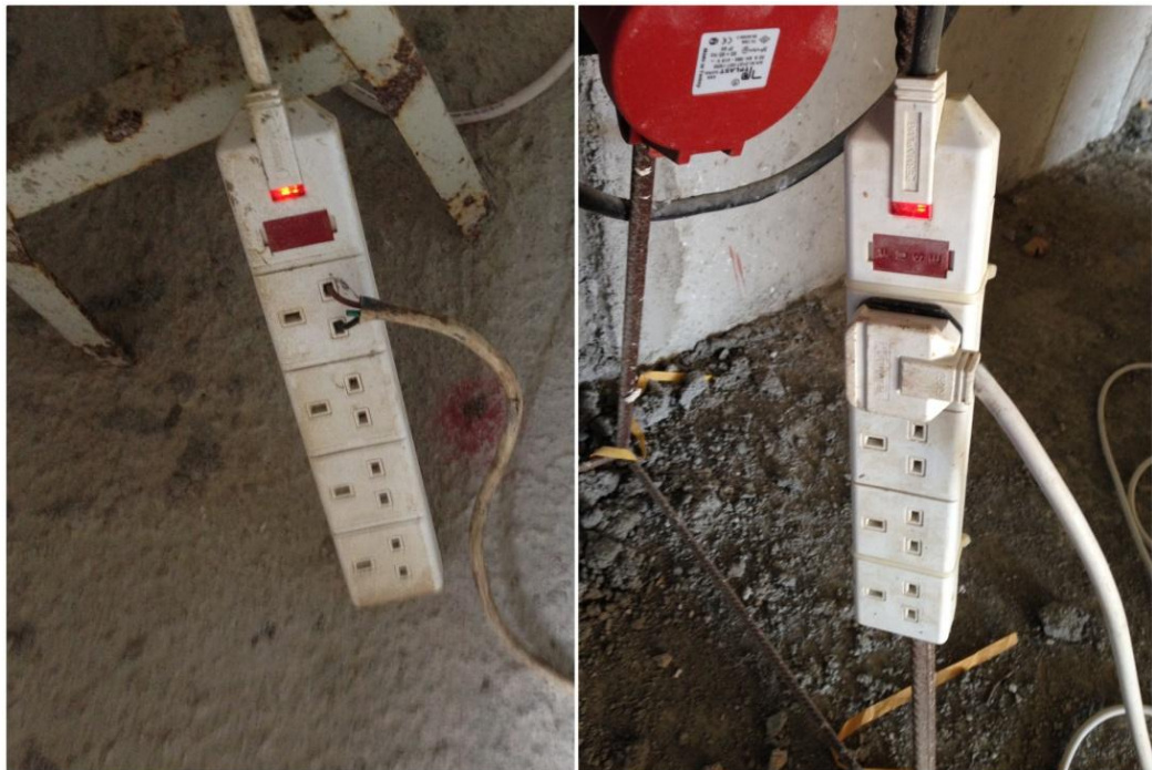
Figure 5.15. Electric extension and socket
