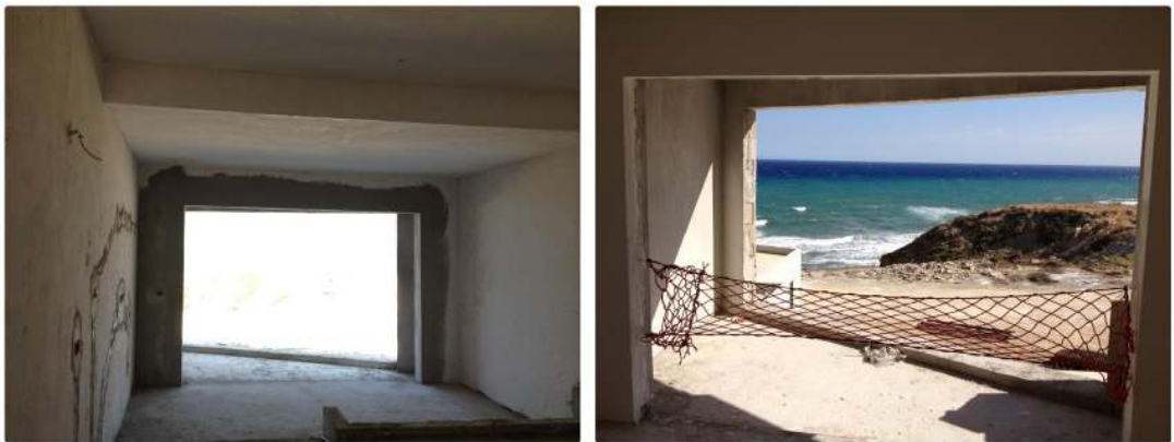
Figure 5.8. Safety net system in LPH project (1)
