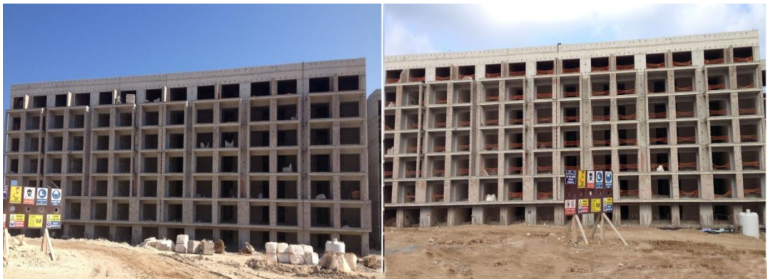
Figure 5.9. Safety net system in LPH project (2)
