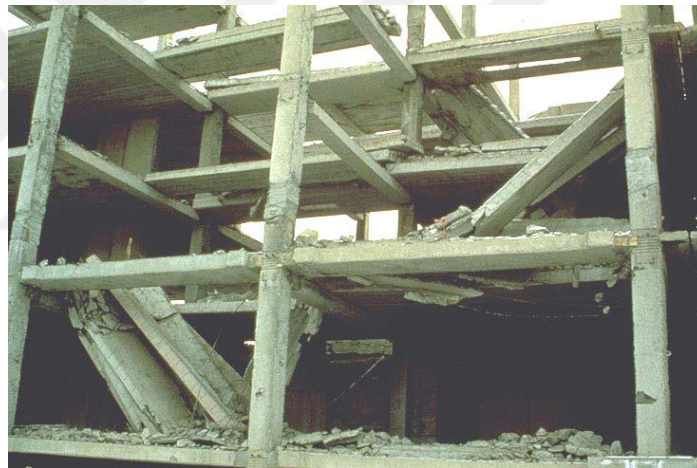
Figure 3.7 Floor plank failure (Clinton, 2009)
