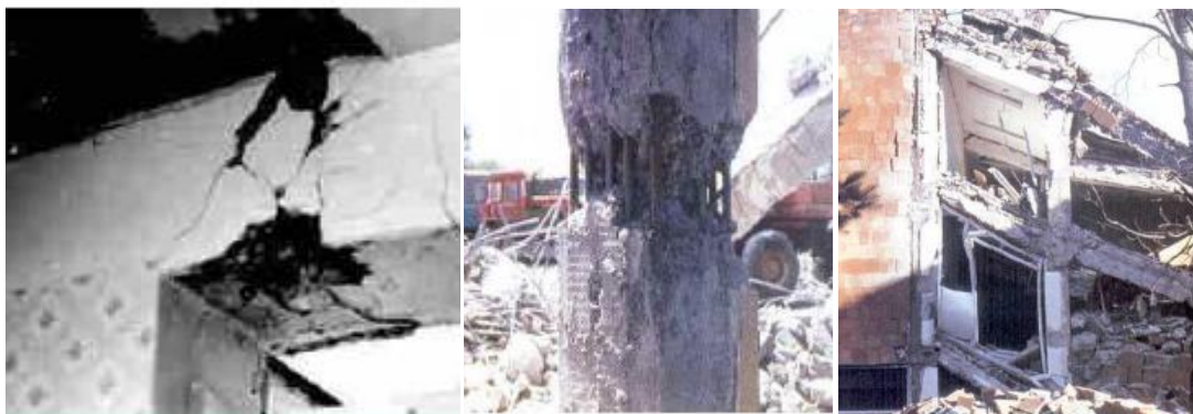
Figure 3.9 Building damage 1988- Armenia Earthquake (Clinton, 2009)
