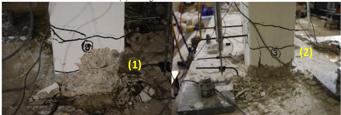
(c) Damage on the column(s) bottom ends
