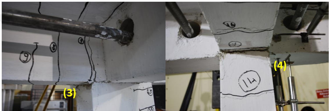
(b) Damage on the beam ends
