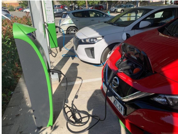
Figure 2.15: Electronic Car Charging System
