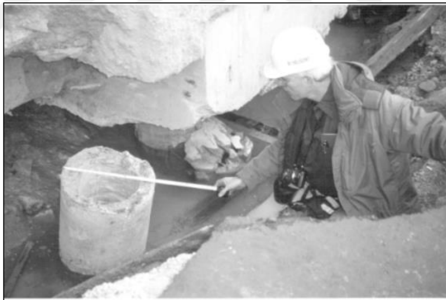
Figure 2.16 Sheared pile due to lateral ground displacement in Kobe Earthquake (1995)
