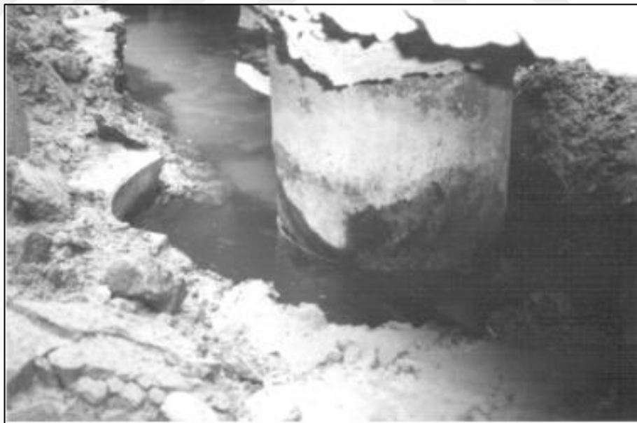
Figure 2.18 Crane rail undamaged piles regardless of the fact that ground lateral displacement more than 1 meter
