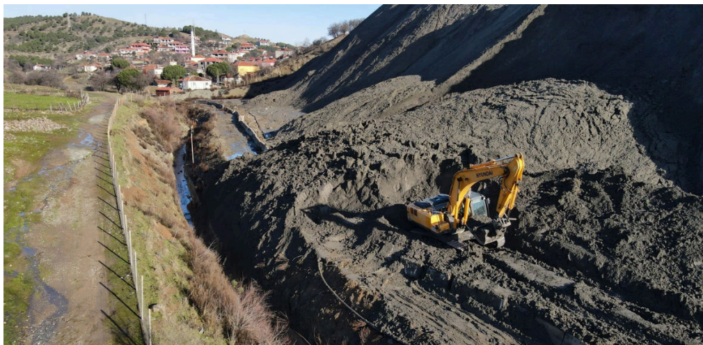
Figure 3.21 A photograph taken after the mine's waste storage collapsed in December 2021 (Politeknik, 2021)
