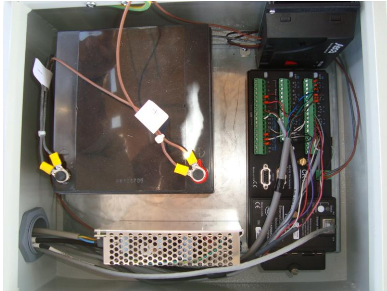
Figure 3.23 The CR1000 Data logger, the NL115 Ethernet module, the power supply, and the backup rechargeable battery that contained in the first enclosure
