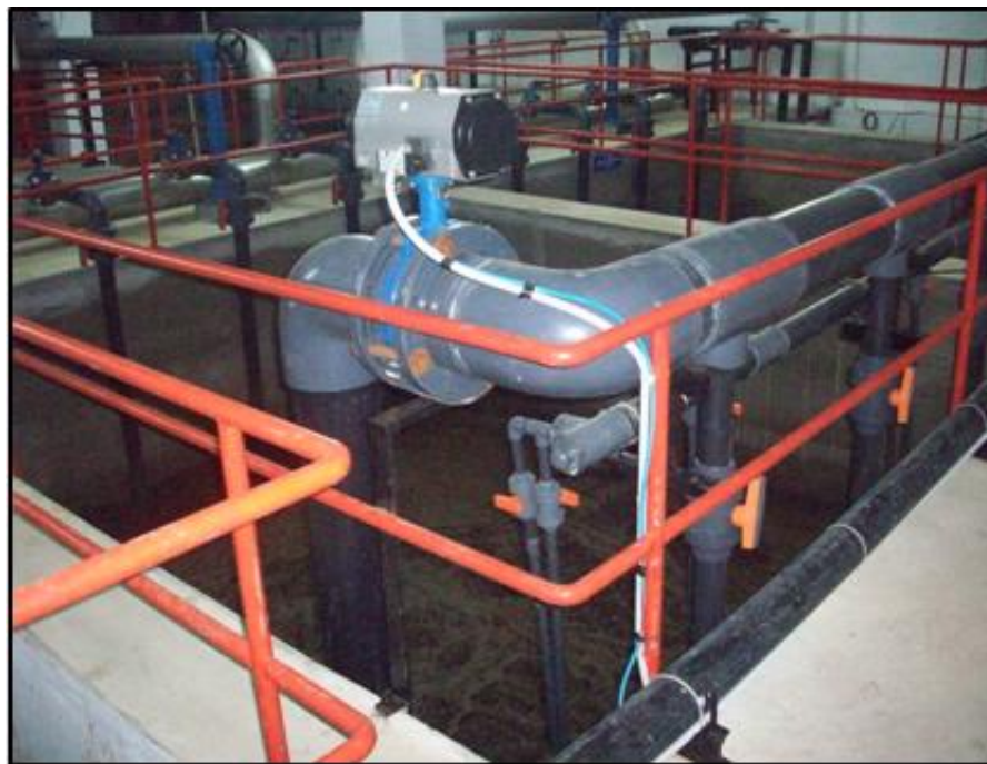
Figure 3.13 MBR automation system
