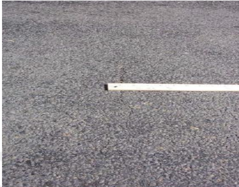
Figure 2.12 Low temperature cracks with low severity (FHWA, 2009)
