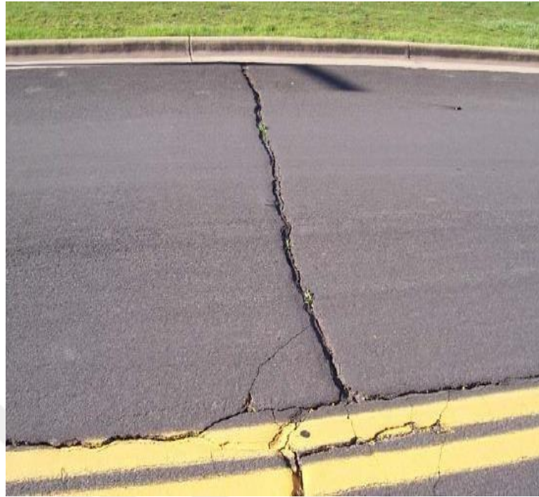
Figure 2.14 Low temperature cracks with high severity (FHWA, 2009)
