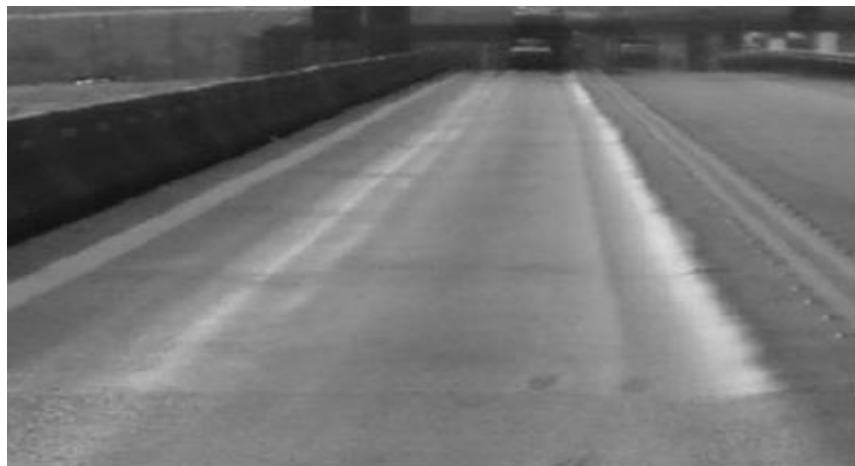
Figure 2.4 Typical rutting quite often formed very early (Nikolaides, 2014)
