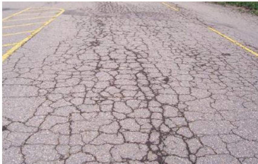
Figure 2.9 Fatigue cracks with high severity (FHWA, 2009)
