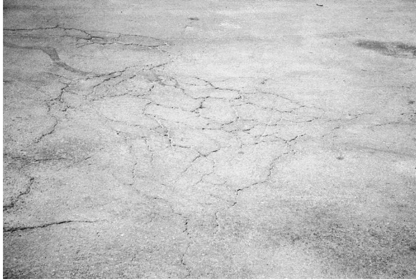
Figure 2.8. Subgrade failure (Lavin, 2003)
