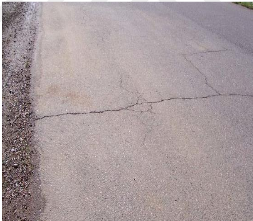
Figure 2.13 Low temperature cracks with medium severity (FHWA, 2009)
