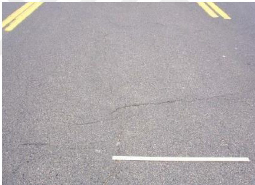
Figure 2.11 Fatigue cracks with low severity (FHWA, 2009)
