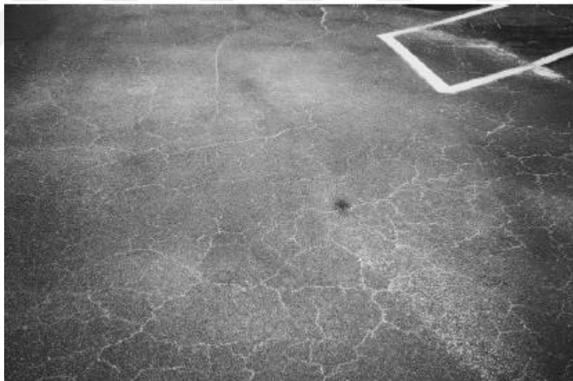
Figure 2.7 Fatigue cracking (Lavin, 2003)
