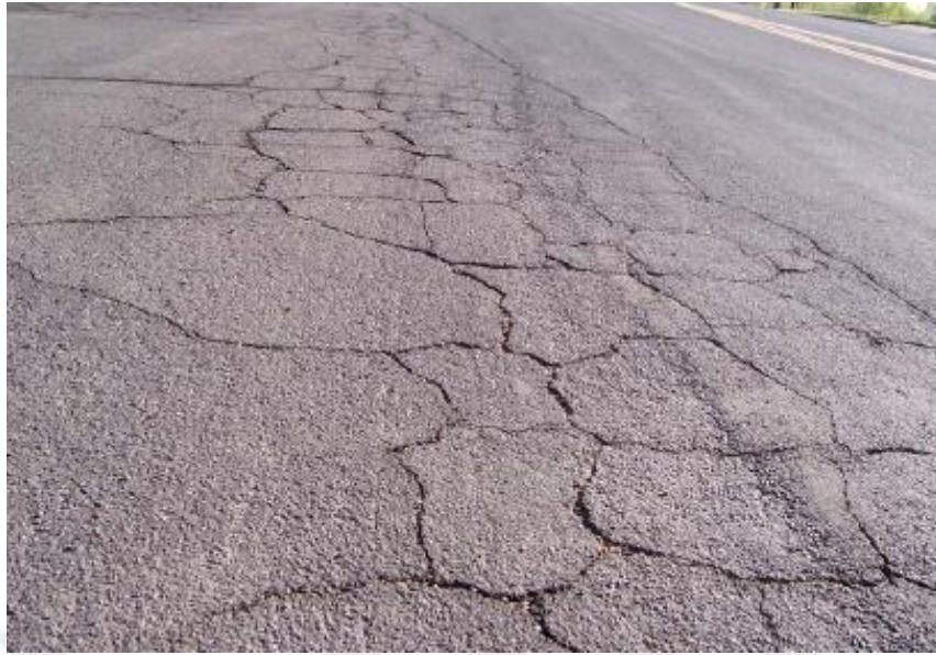
Figure 2.10 Fatigue cracks with medium severity (FHWA, 2009)
