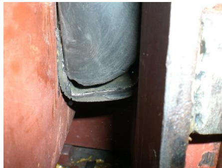
Partially deformed shape of the specimen
