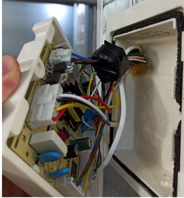
Figure 25: Ferrite Ring (Soft Ferrite) On The Cables in The Control Box
