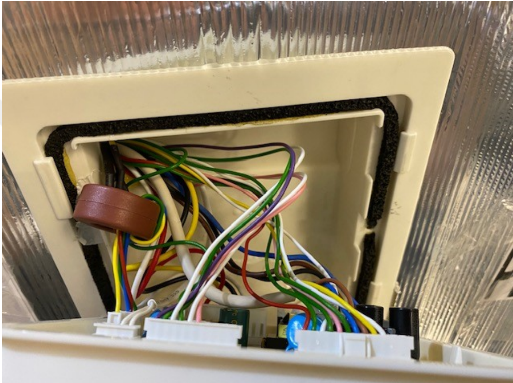
Figure 42: Amorphous core on DC cables
