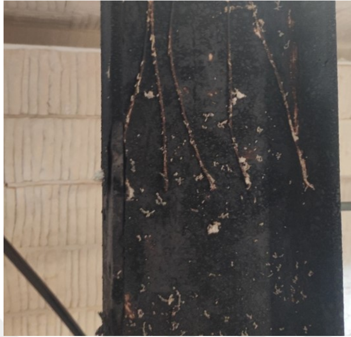
Figure 35: No char on the steel beam which was coated with the Product B
