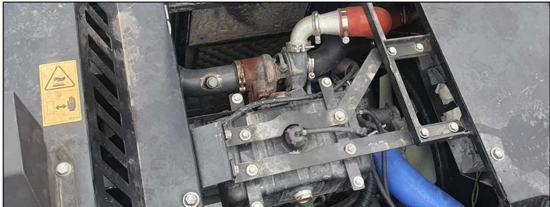
Figure 1: The view of the Diesel Engine
