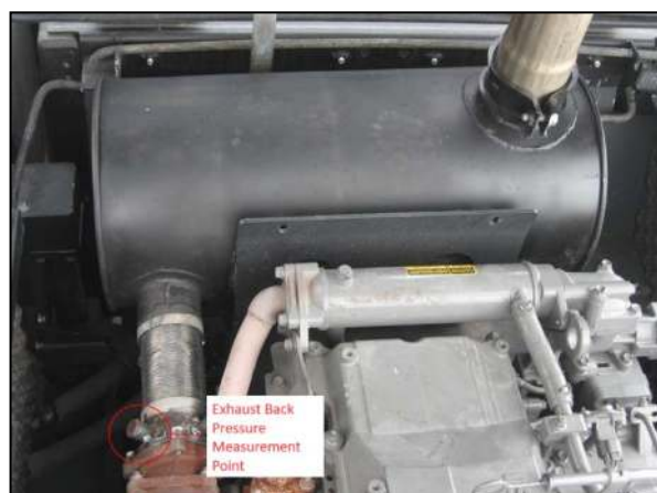
Figure 37: Exhaust Back Pressure Measurement Point
