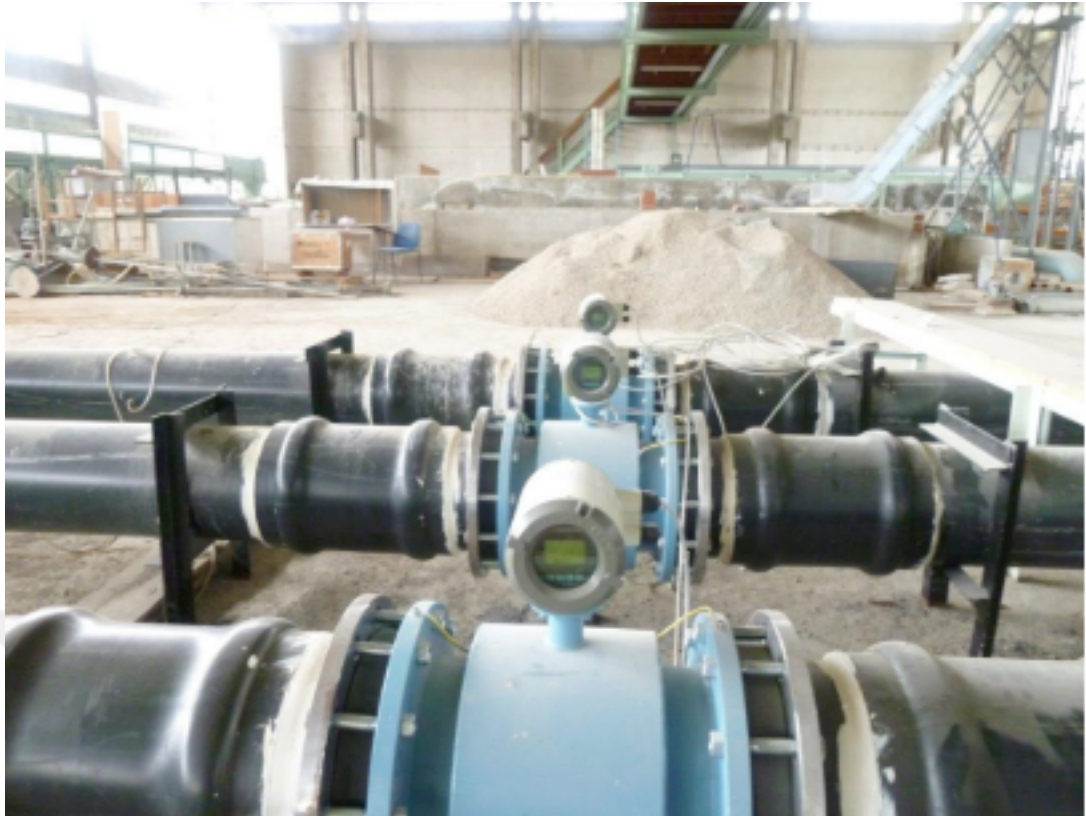
Figure 4.6: Electronic Flowmeters Attached to Downstream of Each Intake
