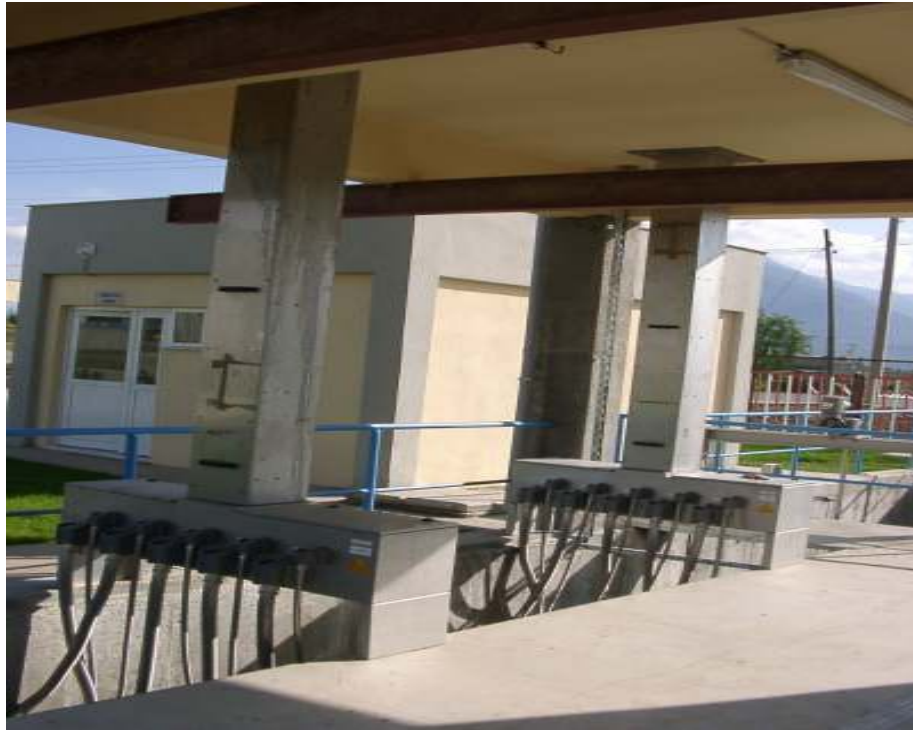
Figure 1.6 Open-channel UV Disinfection System in Fethiye Municipal Wastewater Treatment Plant/Turkey.
