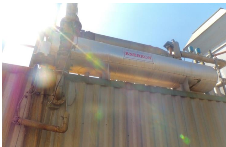
Figure 3.6 Exhaust Gas Heat Exchanger
