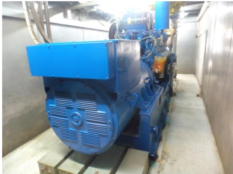
Figure 3.11 DEUTZ Biogas Engine set in cogeneration
