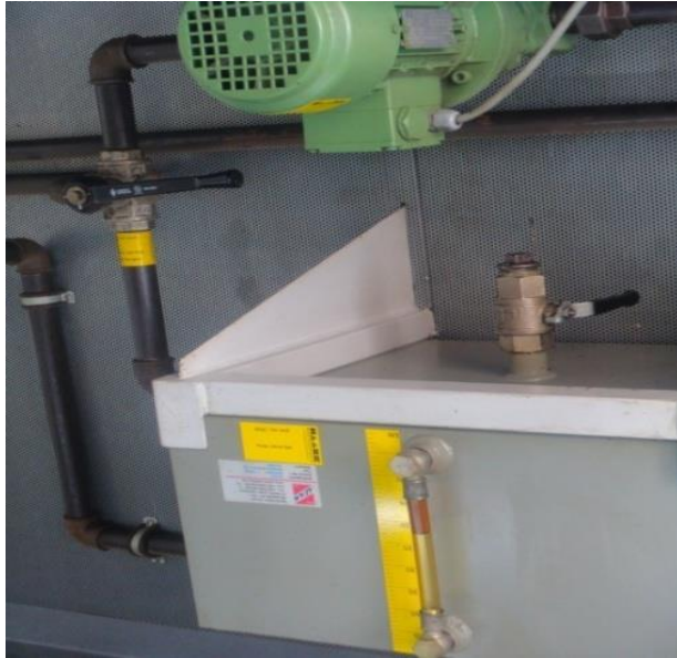
Figure 3.8 Lubrication Oil Heat Exchanger
