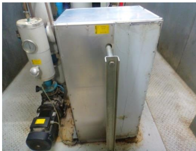
Figure 3.9 Plate Type Heat Exchanger
