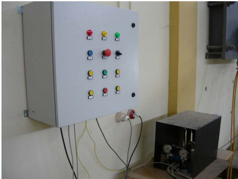
Figure 3.40 Control panel of actuator
