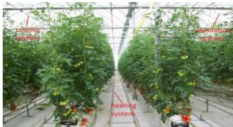
Figure 1.3 Systems in Greenhouse
