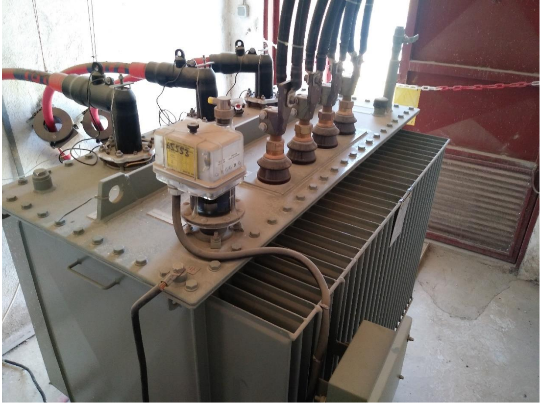
Figure 4.2 Distribution Transformer of AKDENIZ EDAS DS
