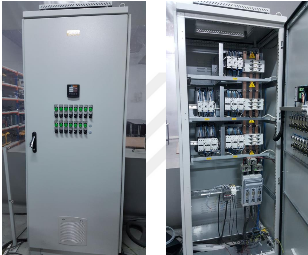
Figure 4.7 100 kVAR Three Phase Capacitive Load Bank
