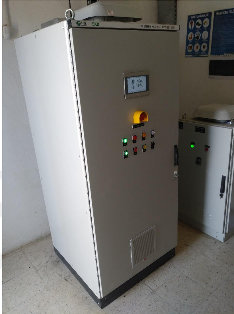
Figure 4.4 EQR Control Panel
