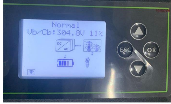
Figure 3.21. Battery Data Hybrid Inverter Screen.
