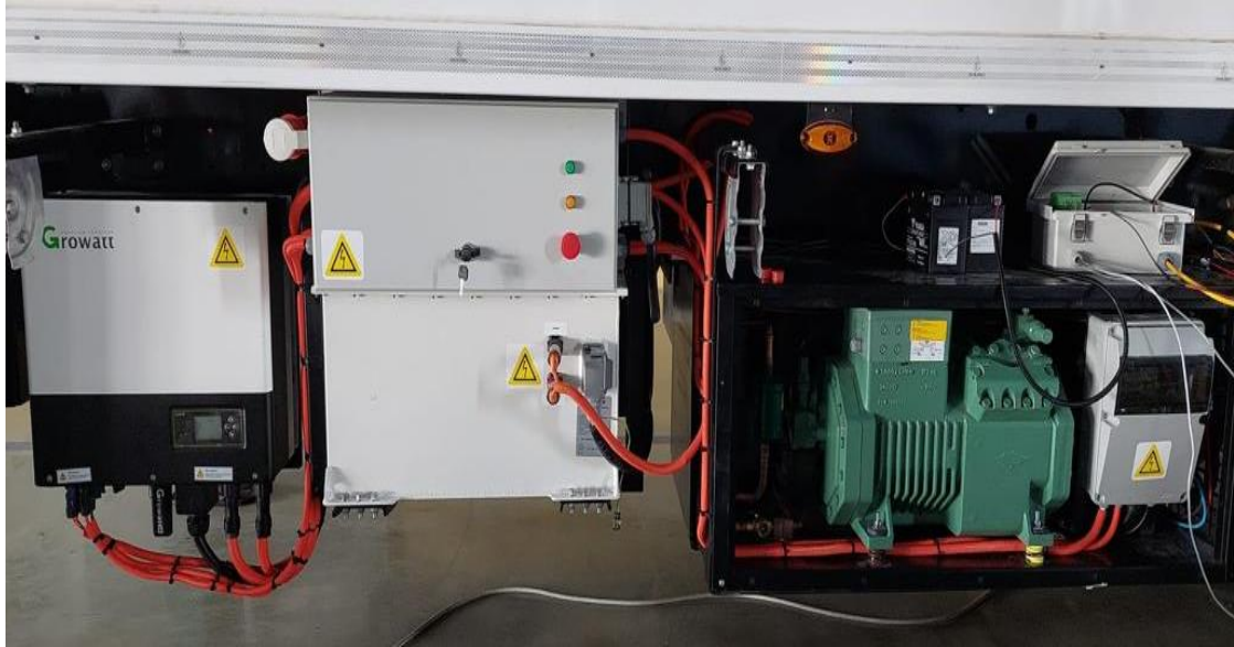
Figure 3.23. Unit Of Energy Storage System.
