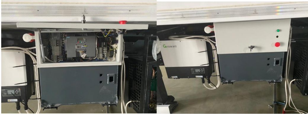
Figure 3.18. Transfer Case And Battery Pack.
