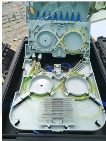
Figure 3.30: Optical Termination Box (OCT).
