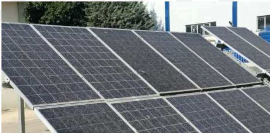
Figure 6.1 six pieces different brand solar panels
