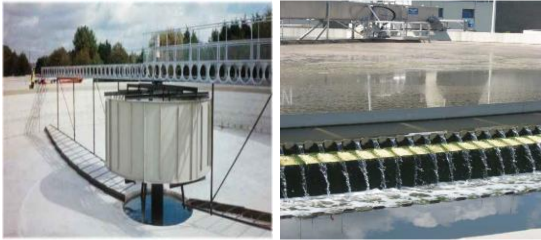
Figure 2.12 Secondary sedimentation tank
