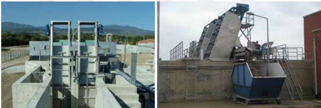
Figure 2.9 Electro mechanic screening system of WWT plant
