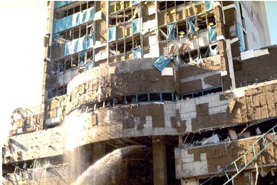
Image 12. On the Day of HSBC Explosion, November 20 th , 2003. This figure shows the damaged HSBC building after the terrorist attack in Levent. (Photo: Reyhan Erkenci).
