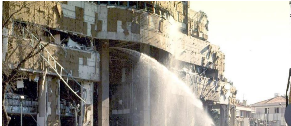
Image 8. On the Day of HSBC Explosion, November 20 th , 2003. This figure shows the situation of the HSBC building in the aftermath of the terrorist attacks. (Photo: Reyhan Erkenci).
