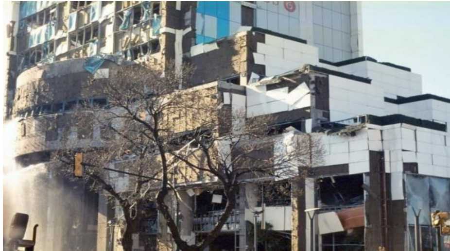
Image 14. On the Day of HSBC Explosion, November 20 th , 2003. This figure shows the damaged HSBC building after the terrorist attack in Levent. (Photo: Reyhan Erkenci).
