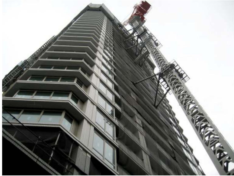
Figure 2.16 The Nabeaure Tower in Yokohoma, Japan uses precast ECC coupling beams in building core for seismic resistance
