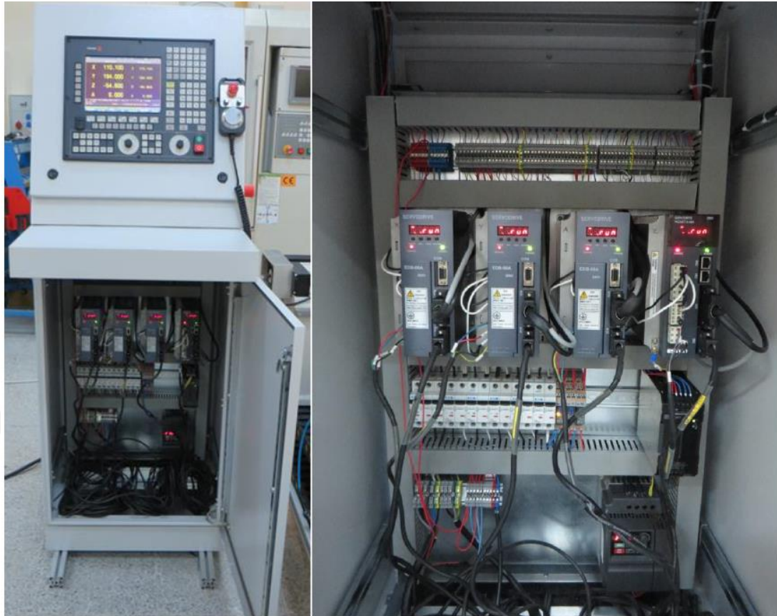
Figure 3.36 CNC control unit and control panel inner views (Personal archive, 2017)
