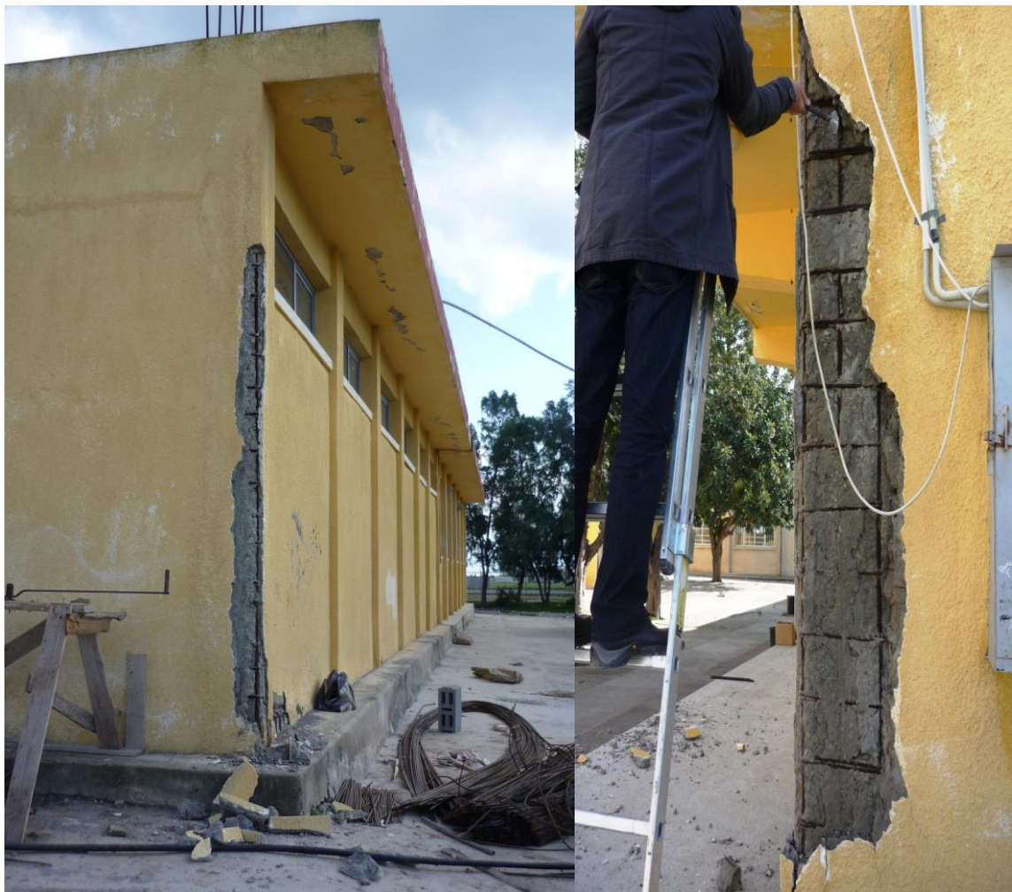
Figure 1.1: Damaged high school building which was demolish (Yalciner et al., 2012a).
