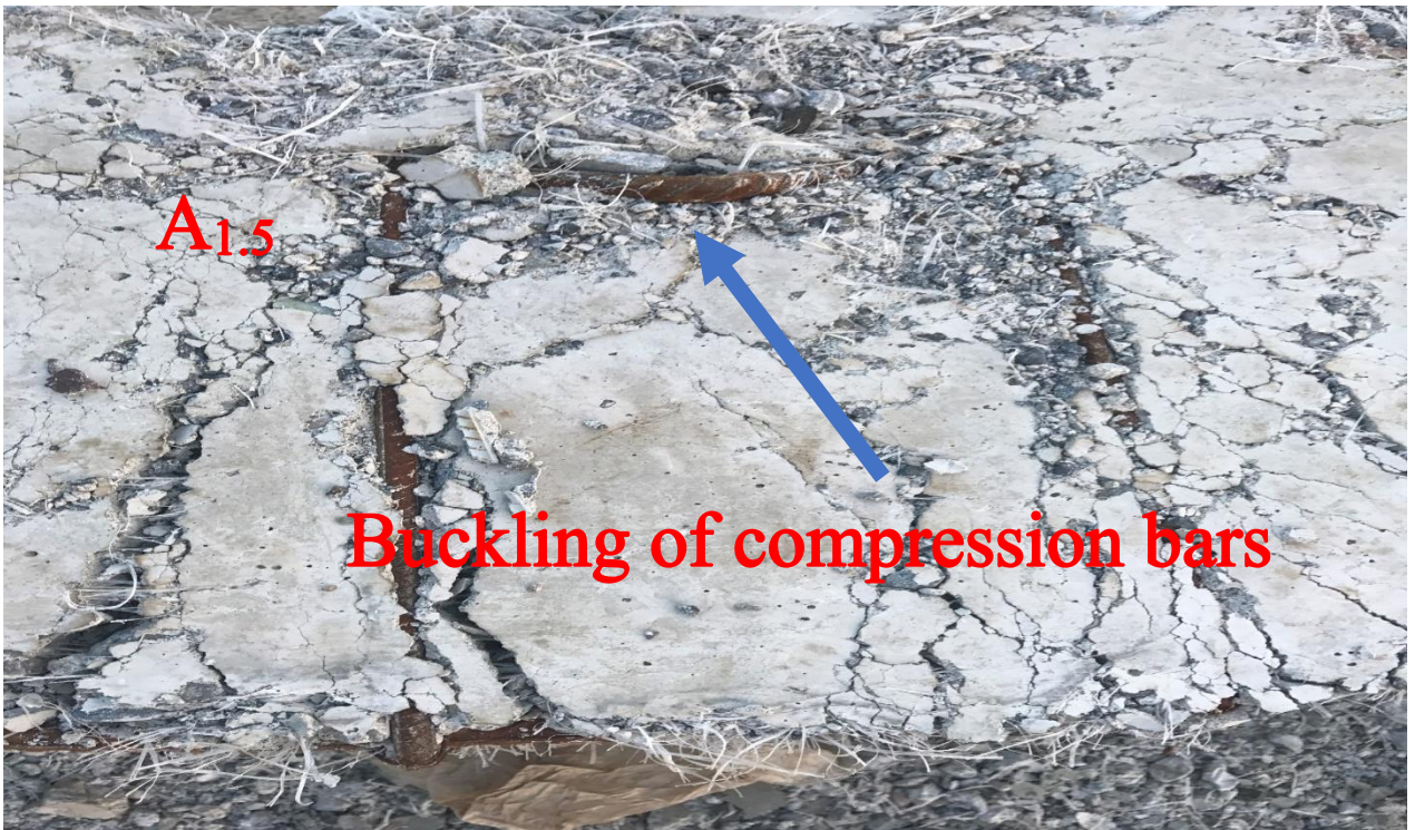
Figure 3. Buckling of compression bars
