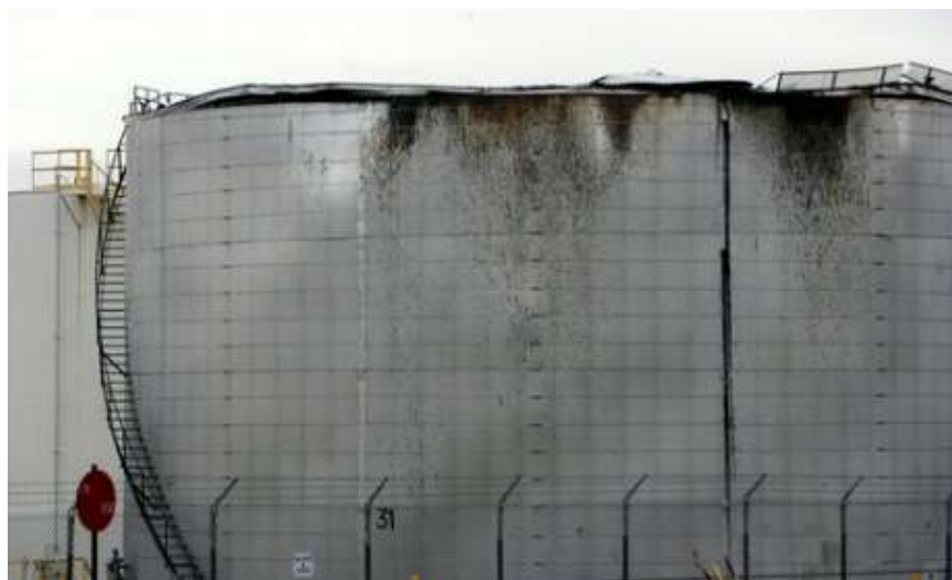
Figure 2.4 Roof damage of storage tank
