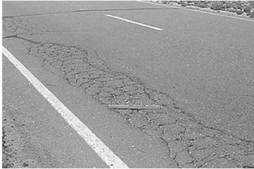
Figure 2.2 Advanced stage of fatigue cracking (Fwa, 2006)
