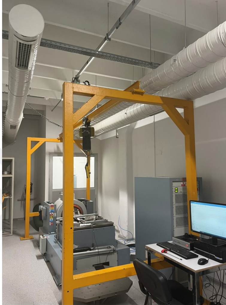
Figure 5: Mechanical Room Ventilation System
