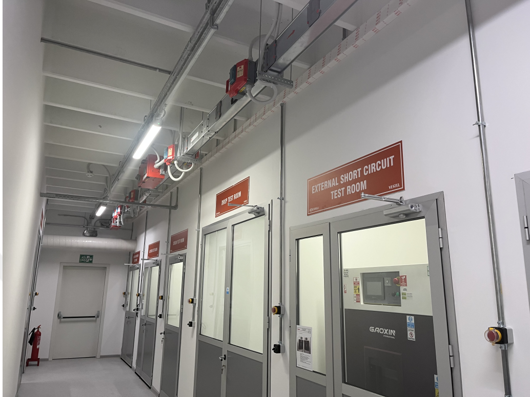
Figure 6: Emergency Stop Buttons for rooms
