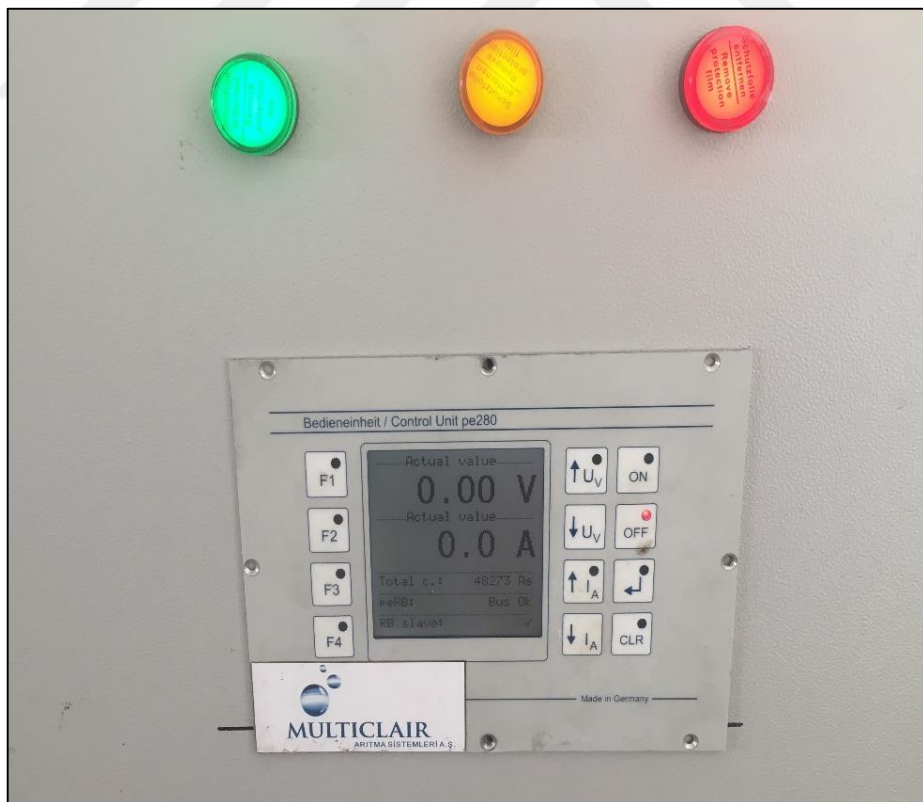
Figure 3.5. E&E process reactor control panel.
