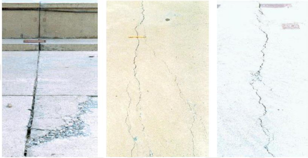
Figure 2.4 SefidRud buttress dam cracks at the crest of the 106 m high (Jaiswal and Jain 2004)
