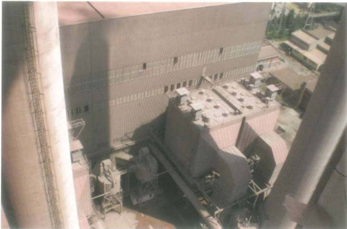
Figure 4.4 Airman plant electro filter
