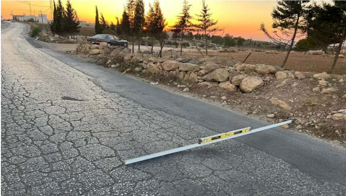
Figure 3.2: Sample for Ruts, Patches, and Cracks.
