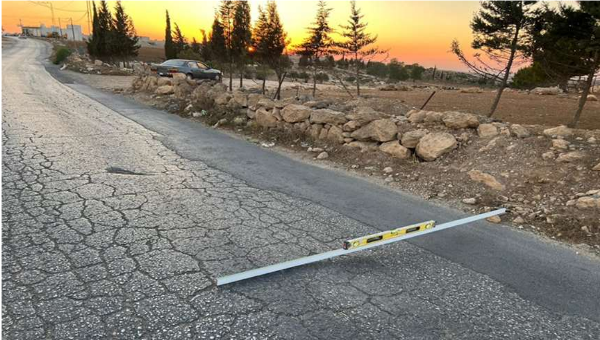
Figure 3.2: Sample for Ruts, Patches, and Cracks.
