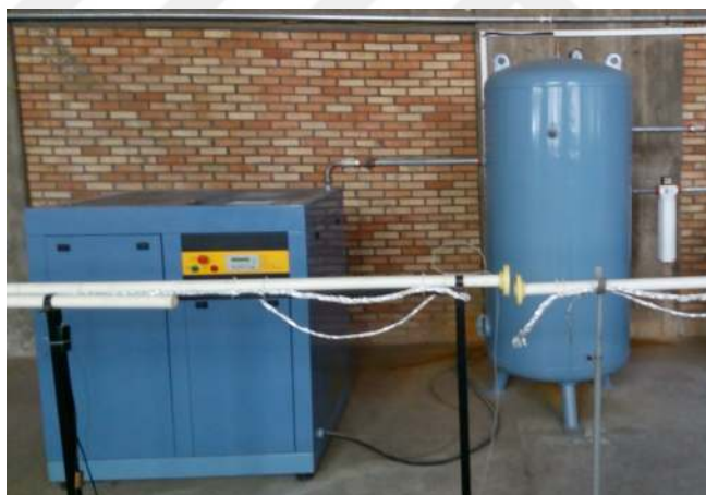
Figure 3.7 Lupamat LKV 30/8 model screw compressor with 1m 3 air tank
