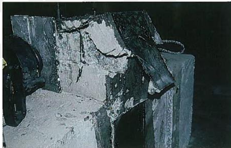
Figure 2.1 Failure of Bracket after fabric cut
