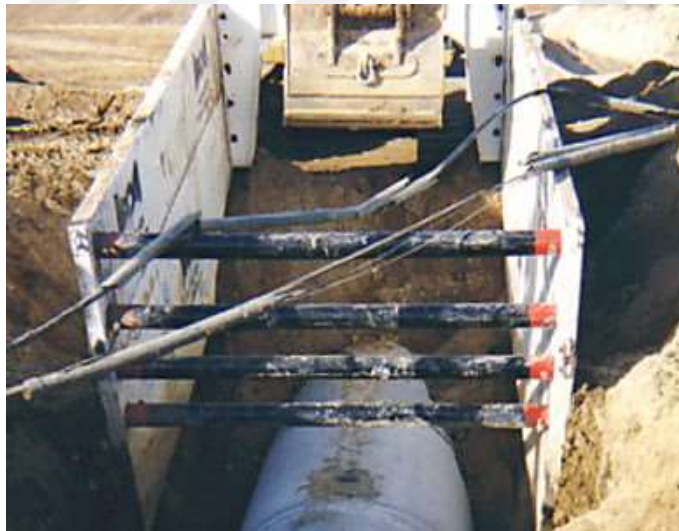
Figure 2.17. Aluminum sheet-pile wall
