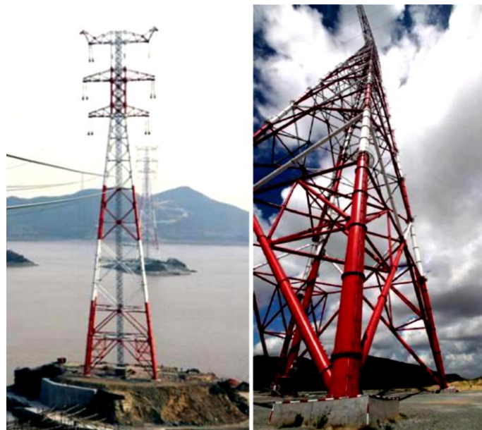
Figure 2.33 Zhoushan electricity tower, China (Huang, 2015)
