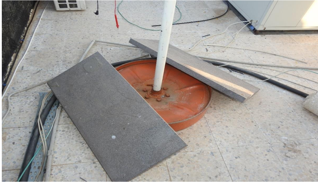
Figure 3.4 Turbine base with additional weight.
