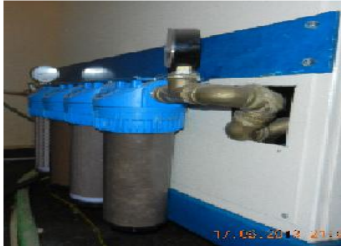
Figure 3.6 Filtration unit with cartridge filters
