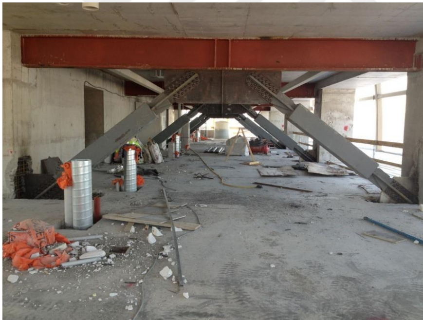
Figure 1.3. Core Brace BRB Application, Folkart Towers, Izmir, Turkey ( Core Brace )
