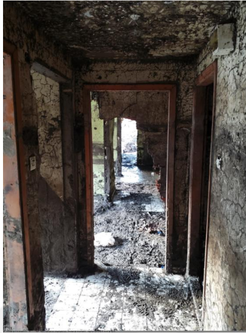
Figure 1-3 Interior damage on a residential building after the 2021 Kastamonu flooding [6]
