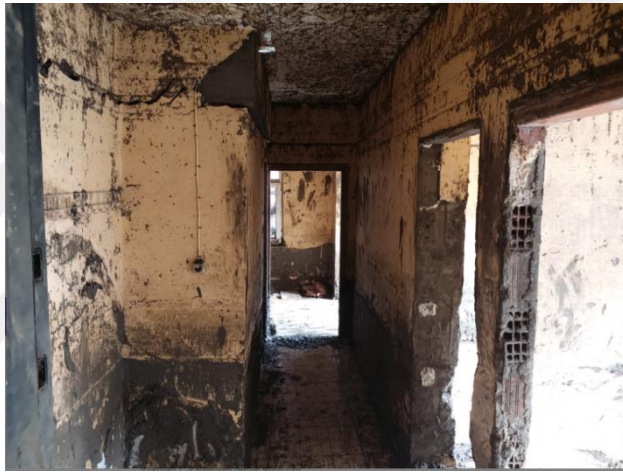
Figure 1-1 Interior damage on a residential building after the 2021 Kastamonu flooding [6]
