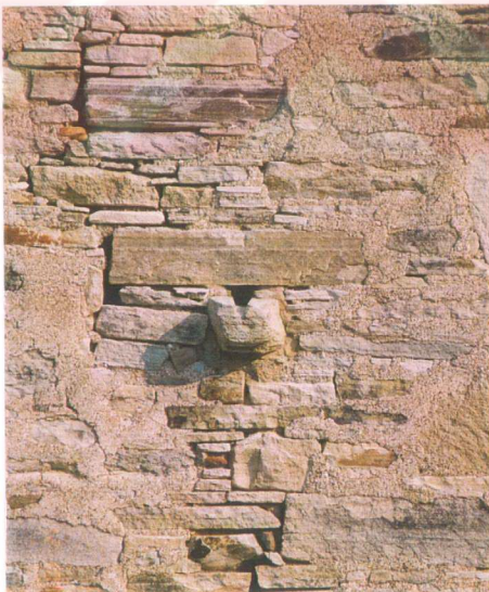
FIGURE.2.126. Drainage Gutter for waste water
