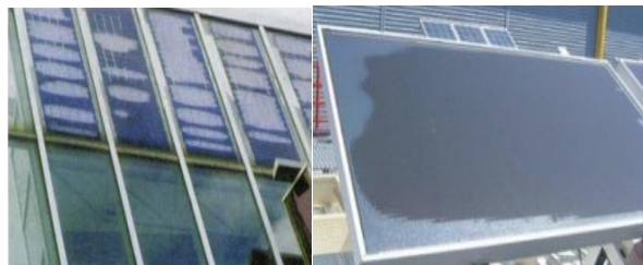
Figure 2.21. Delamination of PV module [80].
