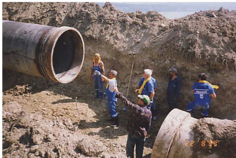
Figure 2.1. Replacement and repair of an axial pullout failure observed in 1999 Kocaeli earthquake (adapted from Ansal et al., 2008).
