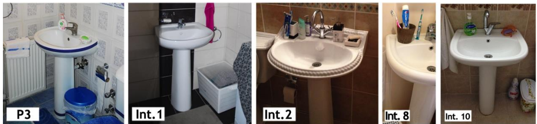
Figure 5.29 : The pedestal washbasins.
